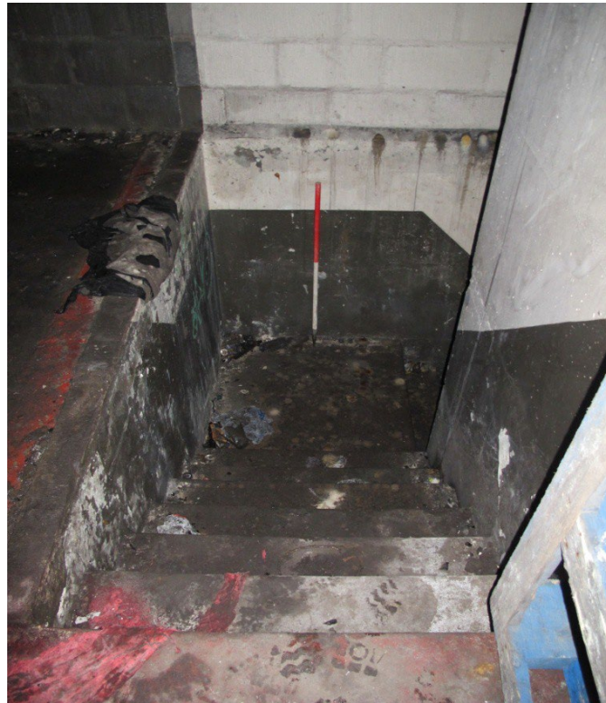
Figure 27: Shot taken of eastern stairwell S3 taken from corridor F4 on the first floor. Looking east.
