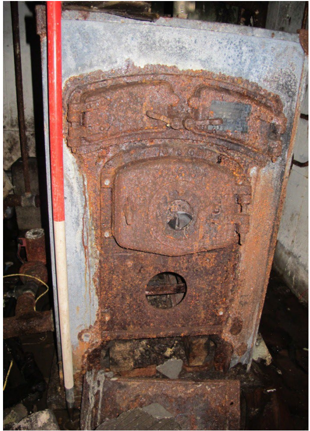
Figure 22: Detail of the cast iron boiler in room G11.
