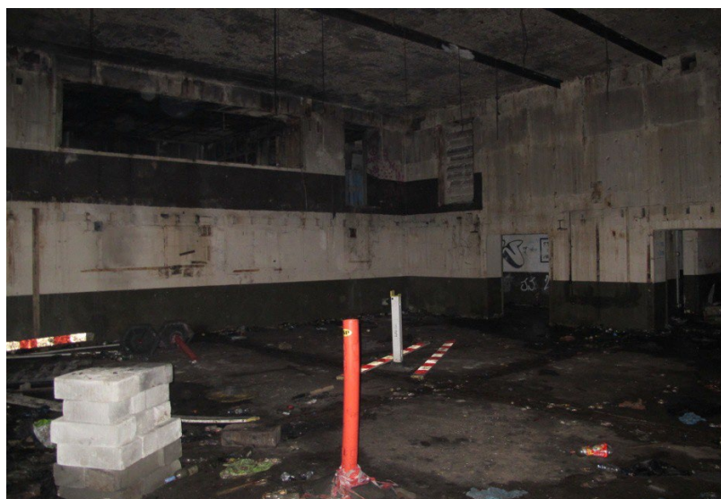
Figure 36: General shot of the main operations room showing the eastern end of corridor F4 terminating with an open doorway on the first floor. Looking northeast.
