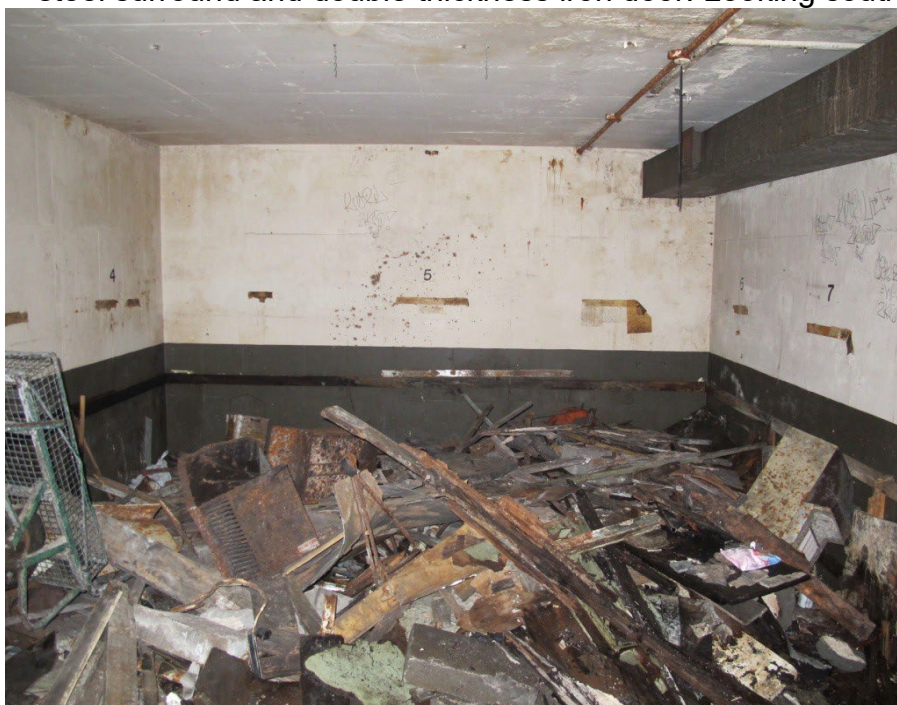
Figure 20: General shot of eastern room G10 partially filled with debris. Looking south.
