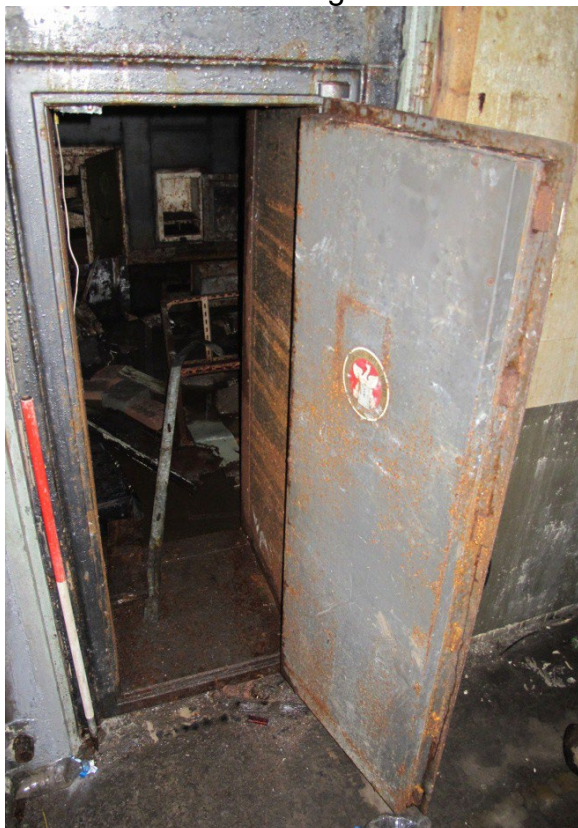
Figure 18: General shot of the safe room G9, showing the three cast iron and steel safes along the south wall. Looking south
