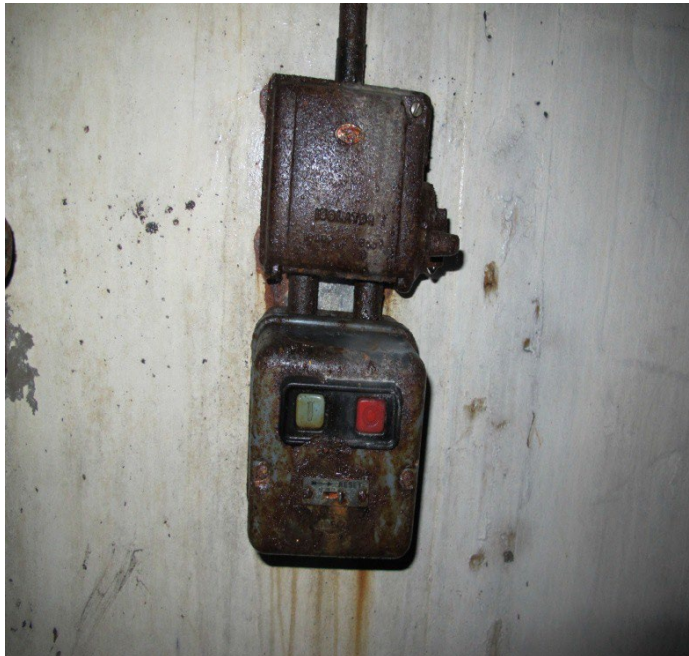
Figure 30: Detail of a power control system mounted on to the south facing wall of room F1. Looking north.
