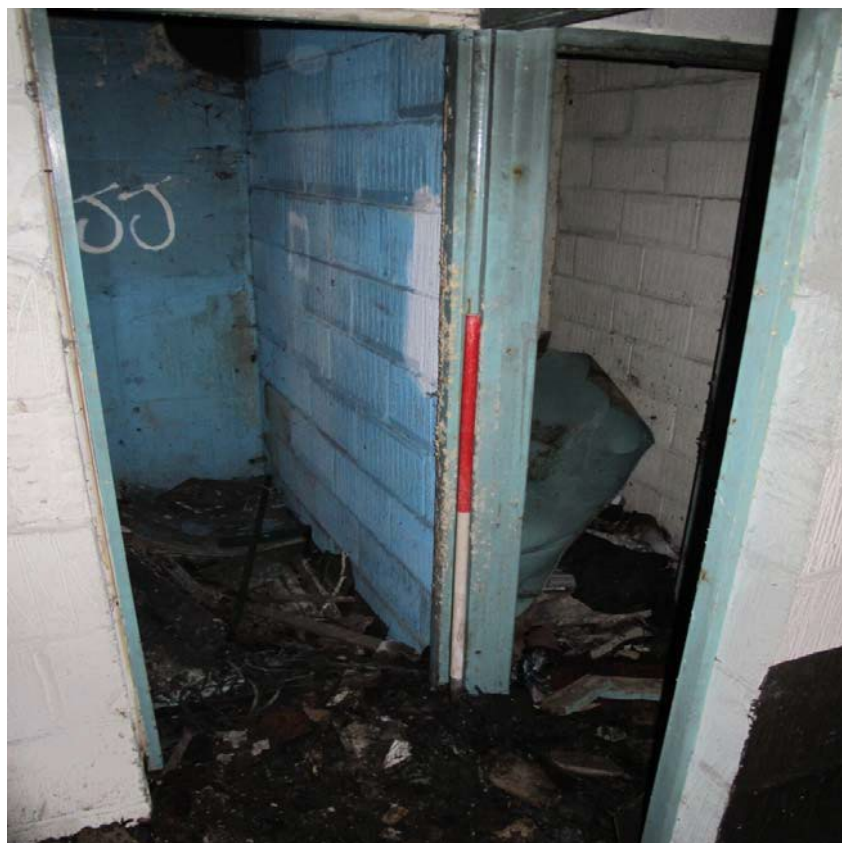
Figure 39: General shot of the breeze block toilet block in north-eastern room F6. Looking northeast.
