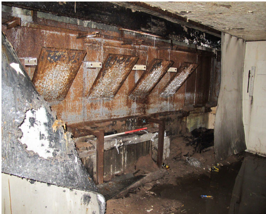
Figure 42: Detail of the butts area behind the damaged target area at the southern end of room F7. Looking southwest.
