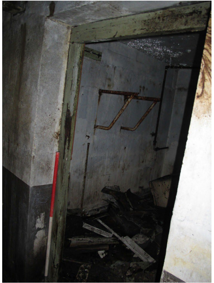
Figure 23: Detail of wall mounted support bars on the west facing wall of room G11.
